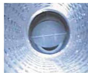
Air duct after cleaning in a hospital
