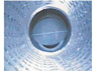
Air duct after cleaning.
