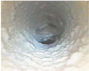
Dirty supply air duct in a hospital.
